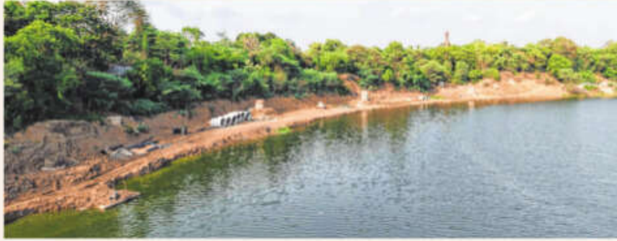
New ghats are being constructed on either side of Kshipra river FP Photos
